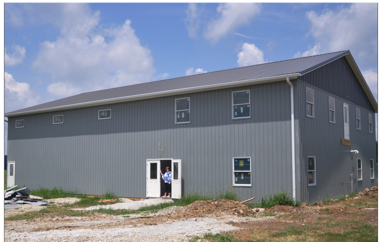
While the building remains under construction, the youth clients at the James B. Wismann Y.E.S. Home will soon have a recreation center thanks to a $100,000 grant from the Lawrenceburg Community Grant Program at DCF.
